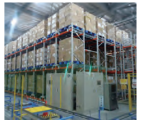
③ High-density storage system
