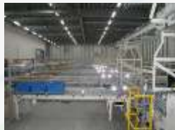
△ Introduce LED lighting
