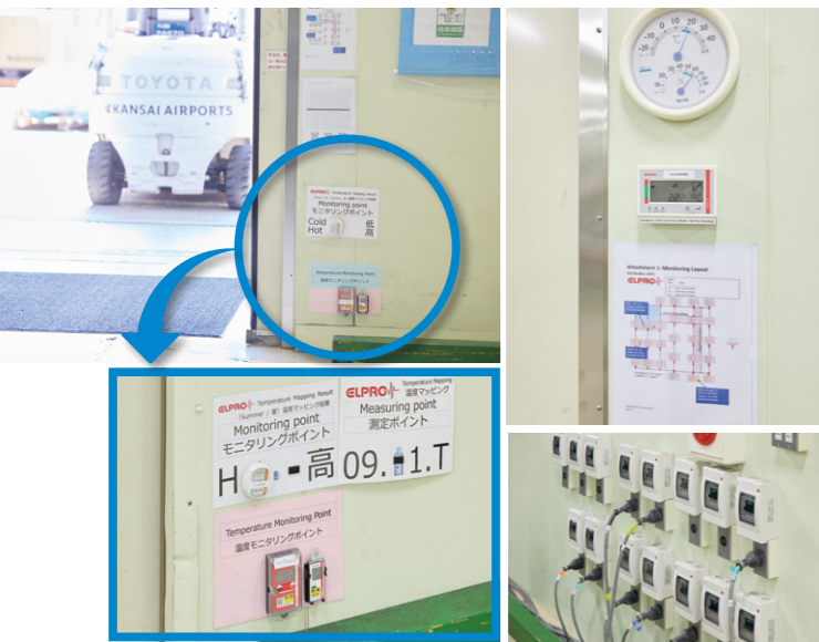
Three photos above: Low-temperature shared cargo terminal at the Kansai International Airport inside KIX Medica. The most important factor in pharmaceutical storage is temperature control. To successfully achieve this, we first check areas that are subject to temperature changes, such as near entranceways. Using these as monitoring points, we check for changes in temperature here. Bottom right: 15 units, compatible with overseas voltage specs, capable of charging rechargeable refrigerated container. System so that voltage does not drop even if all outlets are used at once.
